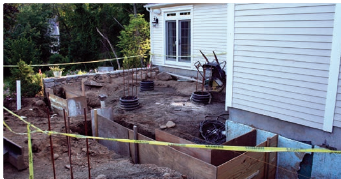
SHOWN HERE: Poor construction led to drainage problems which caused this patio to collapse. The landscape architect corrected the problem by excavating below the basement floor level. Crushed footing drains and septic piping were replaced and a drainage mat was installed against the foundation. New backfill material was distributed and compacted in lifts to allow concrete caissons to rest on undisturbed grade providing a solid support for the concrete patio slabs.
